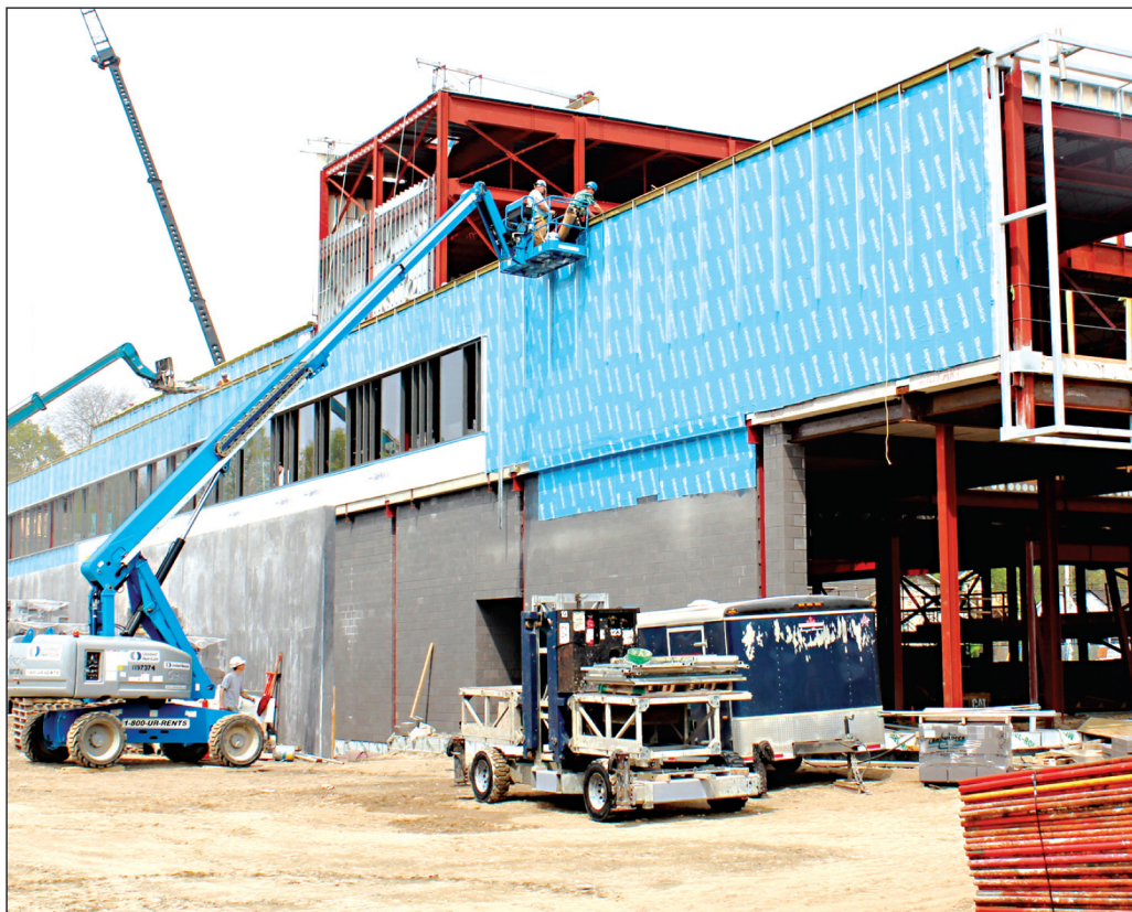
DUNFIELD RISING: Construction continues on the new theatre complex in west Galt while an announcement at the Cambridge Chamber of Commerce Monday morning stated that Shiplake Management, which owns the Dunfield Retirement Residence currently being built in the city, purchased exclusive naming rights for the next 25 years for $1 million. The theatre will be named Dunfield Theatre Cambridge.
